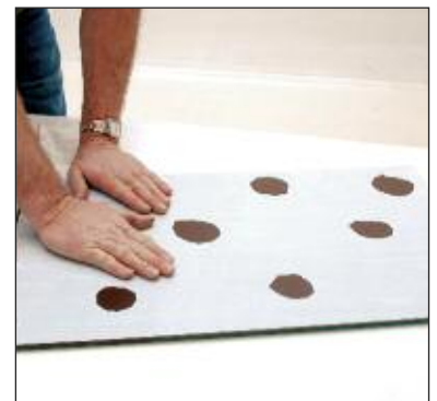
Tape applied to back with holes cut out for application of mastic. Application temperature range is 60 to 100°F (15 to 37°C).
