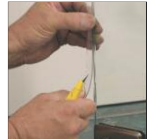
Cut the new and matching water seals to the same length as the originals and install.
